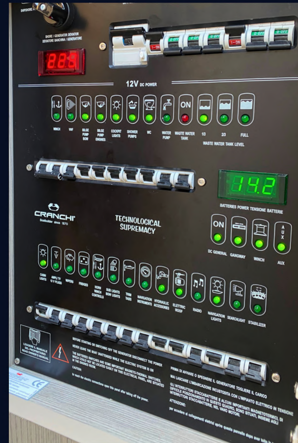
Main Circuit Board
